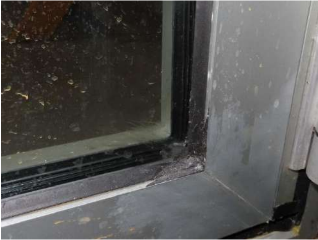
Picture 19 External glazing seal
